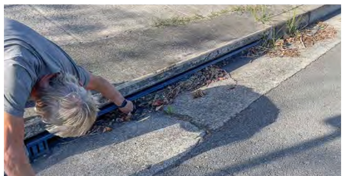
We found many of the street curb inlets debris screens around Keolu Drive were in need of cleaning and repair by the city.
